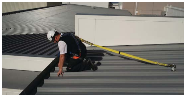
Fall restraint using roof anchor
