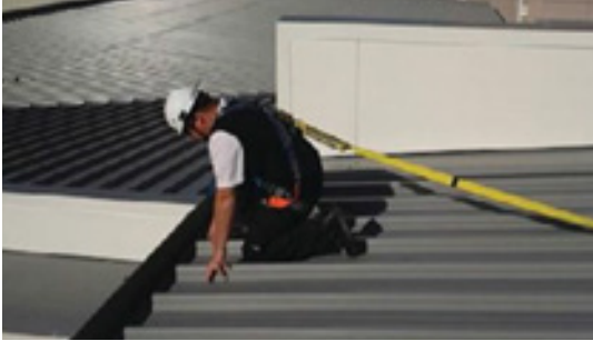
Fall restraint using roof anchor
