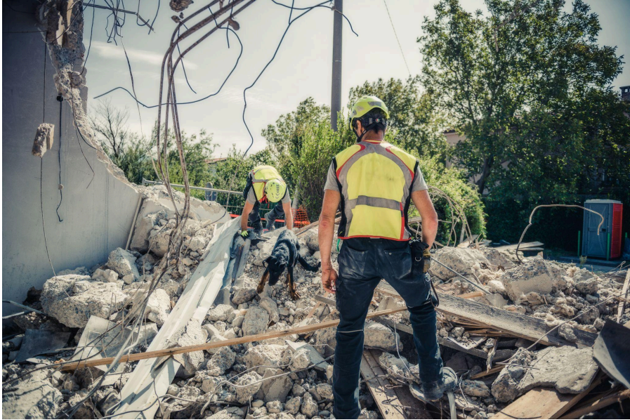
Crews search through rubble
